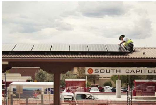
A trainee in the Green Collar Pre-Apprenticeship program installs a solar panel
